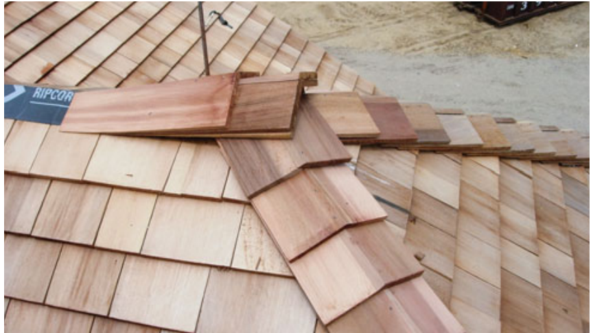
Figure 9. The author buys these made-to-order hip and ridge caps through his roofing supplier, greatly speeding installation. A strip of self-adhering membrane adds another layer of protection under the cap.
