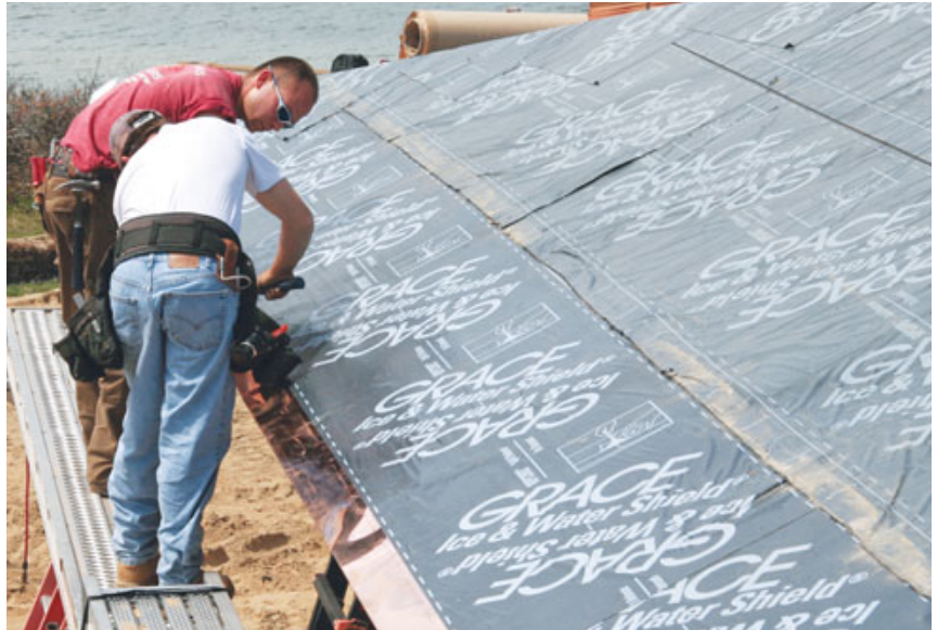
Figure 2. On this waterfront roof, the builder covered the entire roof with self-adhering membrane, eliminating the use of standard #30 felt underlayment. With a self-adhering membrane and reduced course exposure, cedar shingles may be installed on roof slopes as shallow as 3/12.
